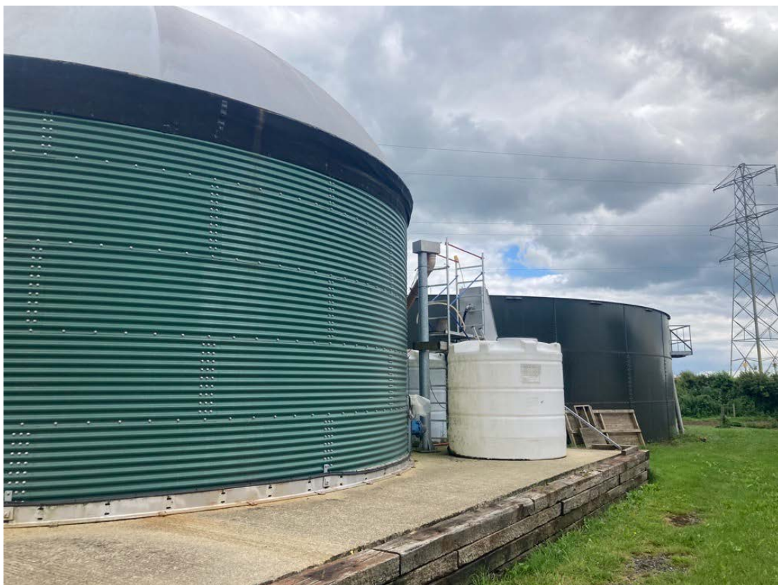
Figure 4. Biogas Plant in a farm. Courtesy of Cecilia Burnfield (CKIC) and Bioplex
